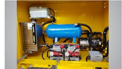
HEATING SYSTEM FOR LUBE OIL TANK
