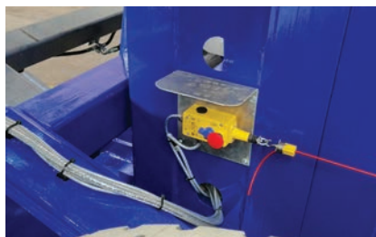
Emergency pull cords
