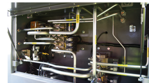
Steel pipework for better heat dissipation
